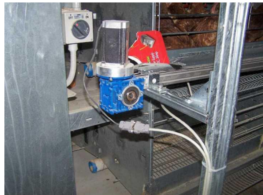
Figure 1. The drive motor for the robot installed at DPI Werribee.
