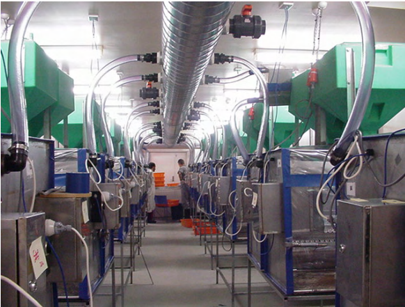
Plate 2. Interior of isolator facility at UNE showing 24 isolators and main air inlet duct. This carries HEPA filtered, heated air to each isolator. Note the green feed hopper above each isolator.
