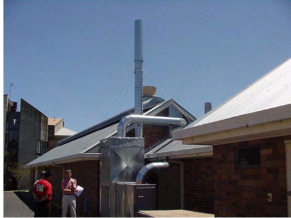
Plate 3. Exterior of the isolator facility at UNE showing the plant room on the right and the main isolator facility in the middle with the air extraction and filtration system next to the people.
