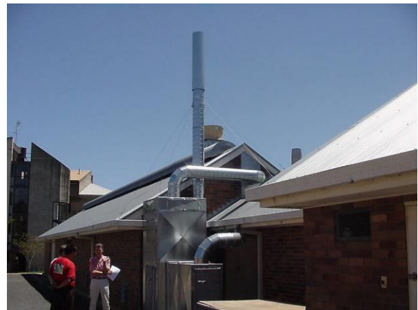
Figure 1-3: Exterior of the isolator facility at UNE showing the plant room on the right and the main isolator facility in the middle with the air extraction and filtration system next to the people.
