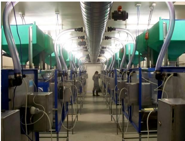
Figure 1-2: Interior of isolator facility at UNE showing 24 isolators and main air inlet duct. This carries HEPA filtered, heated air to each isolator. Note the green feed hopper above each isolator.
